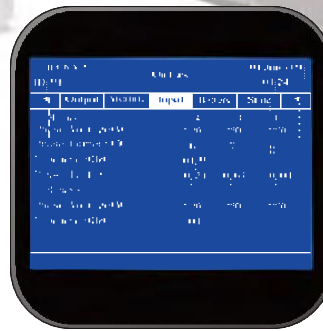
UPS Cabinet Control Panel
