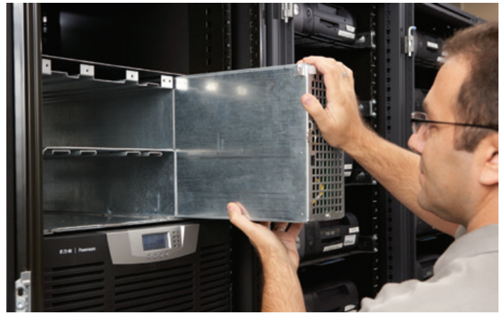
IT staff can easily install electronics modules.
